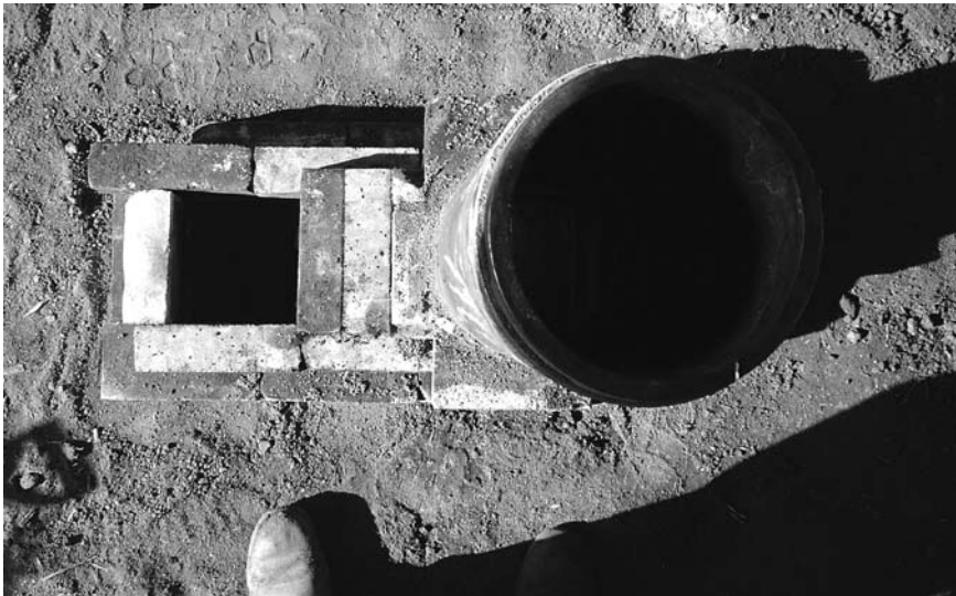
Looking down the barrels of the feed tube and heat riser.
