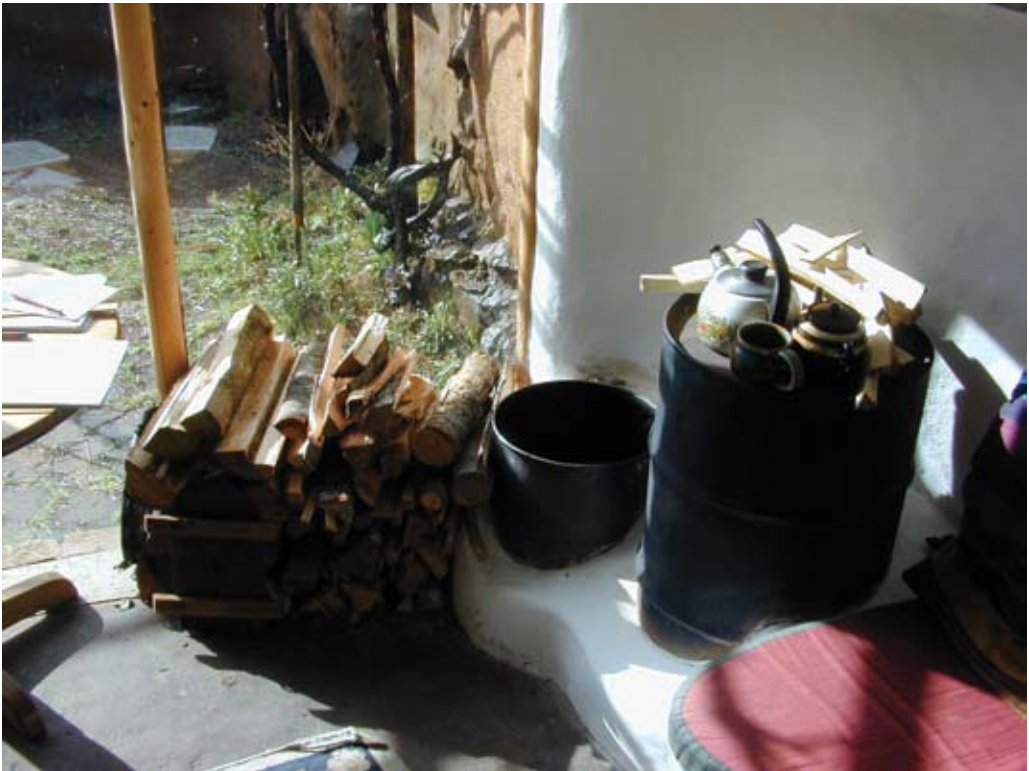
Above: The Rocket Mass Heater with bench at lower right in the home of Ianto Evans and Linda Smiley has been in use for over ten years. Dry firewood, split thin and cued up in the sun, small feed barrel and heat exchange barrel nestled in cob.
