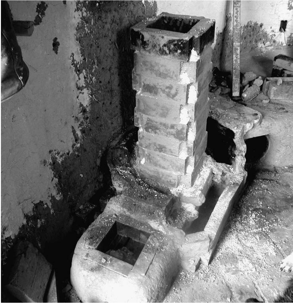
A good example of a brick tower under construction in Chris and Jenn Reinhart's house. A fortress of brick is mortared in to support the barrel. Photos, this page: Chris Reinhart.
