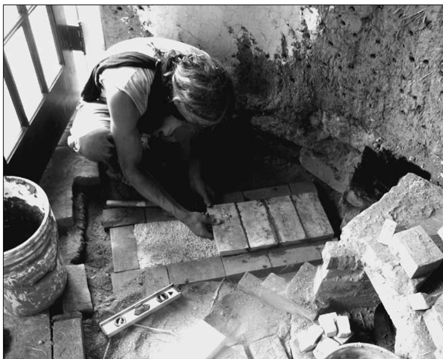
Chris laying the foundation for the stove. The burn tunnel of brick rests on a bed of perlite. Note Chris is building his first layer of brick and insulation sub-floor level. You can see the completed stove on page 84. Photos, this page, Christopher Reinhart.
